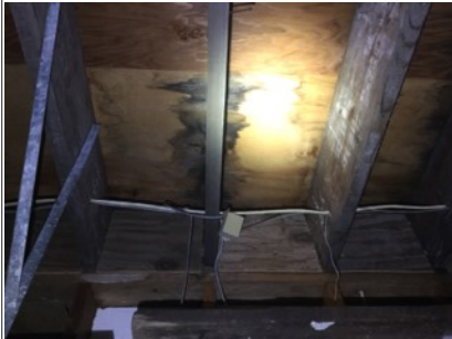
Moisture staining in the garage ceiling. Didn't appear to be active at the time of inspection. Recommend monitoring and repair as needed
