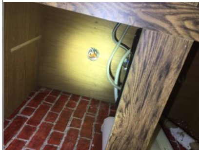
Junction box under the kitchen sink needs a cover. -safety issue
