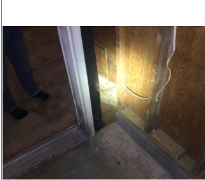
Missing fire rated separation wall between garage and living space. -potential safety issue
