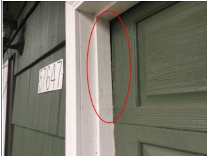
Missing weather stripping
