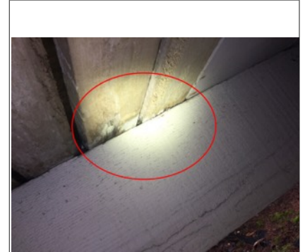
Wood walks and deck flooring has some moisture damage/rot. Recommend further evaluation and repair by a qualified contractor
