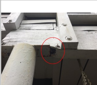
Recommend repairing rotted wood on exterior walk to laundry room
