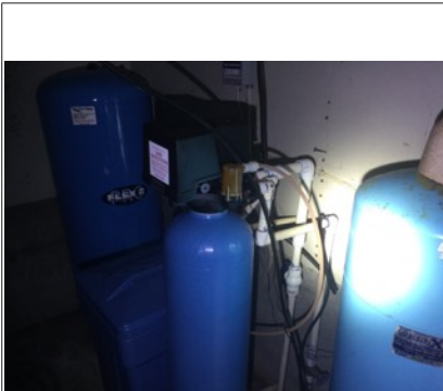
Recommend inquiring with the sellers about the water softener maintenance. Sulfur smell on the interior possible due to maintenance needed
