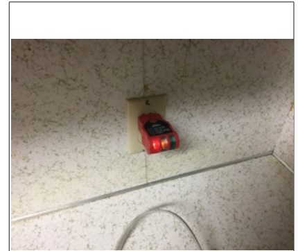
Reversed polarity and no overload GFCI protection in the basement kitchen within 6 feet of the sink. Safety issue
