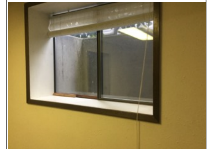
It is estimated that at some point moisture may make its way through most basement floors me/or walls. Recommend monitoring
