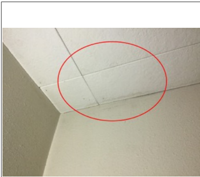
Moisture staining in the ceiling
