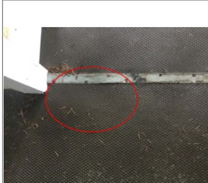
Recommend repairing rotted wood flooring where the walk meets the deck.
