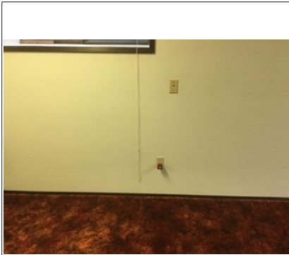
Open ground in the bonus room near the kitchen. -safety hazard
