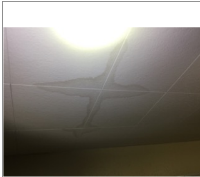
Moisture staining under the washing machine. Recommend drip tray be installed under washing machine
