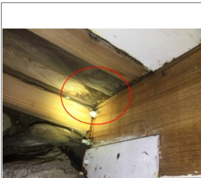
Recommend replacing rotted wood on deck/walks
