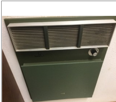
Heaters in bathrooms were in marginal condition.
