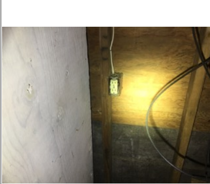
Missing outlet covers and no overload GFCI protection in the garage. -safety issue
